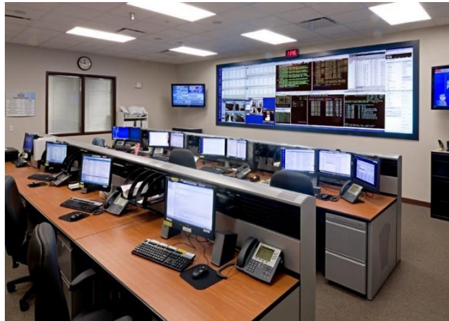
Gambar 52 : Control Room Data Center
